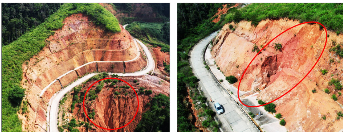
Figure 1. Erosion damage worsening in Kon Tum, Vietnam [8]
