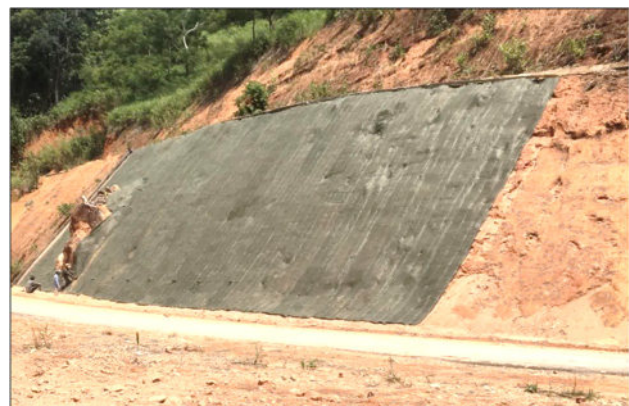
Figure 12. Complete installation in August 2022 [3]
