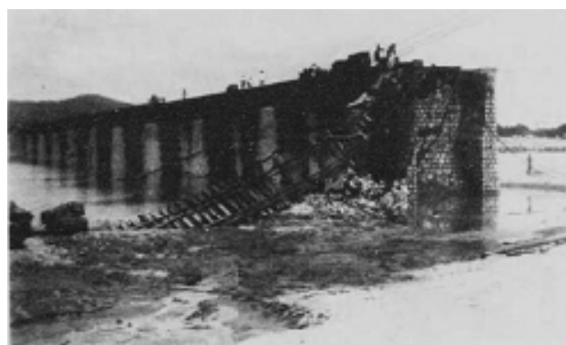
Figure 4. Failure of Han River Railway Bridge in July 1925. (Japanese Government - General of Korean Peninsula, 1926)
