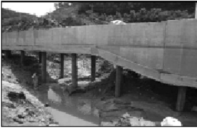
Figure 9. Failure of a levee around drainage conduit.
